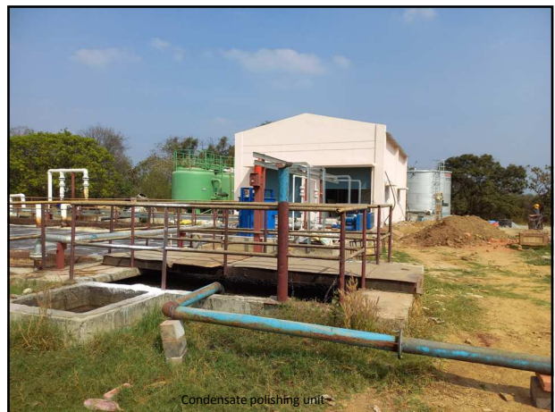
Condensate polishing unit
